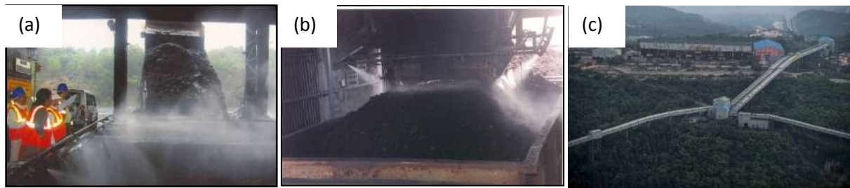
Figure 9: Fully enclosed Coal Handling Plants at NCL: Mist Spray Dust Suppression System at (a) gyratory crusher point, (b) Rapid Loading System of Silo and (c) bird eye view of CHP at NCL
