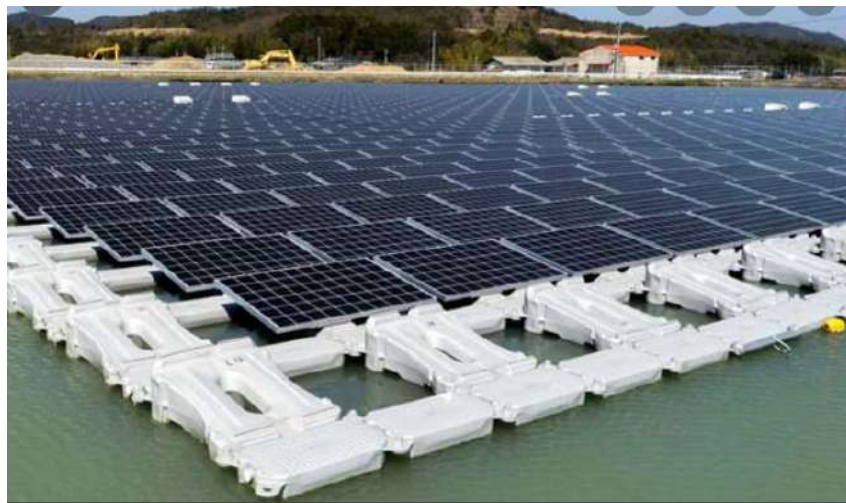
Figure 2- Showing floating Solar panels mounted on galvanized steel
